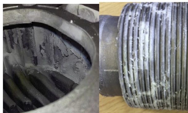
Fig. 11. Silica deposition in the aluminium heat exchanger of appliance 6 after roughly 1050 h of operation 11.2 \text{ mg Si/m}^3 in the fuel. Left: top of the heat exchanger; right: bottom insert in condensing part of the heat exchanger.
