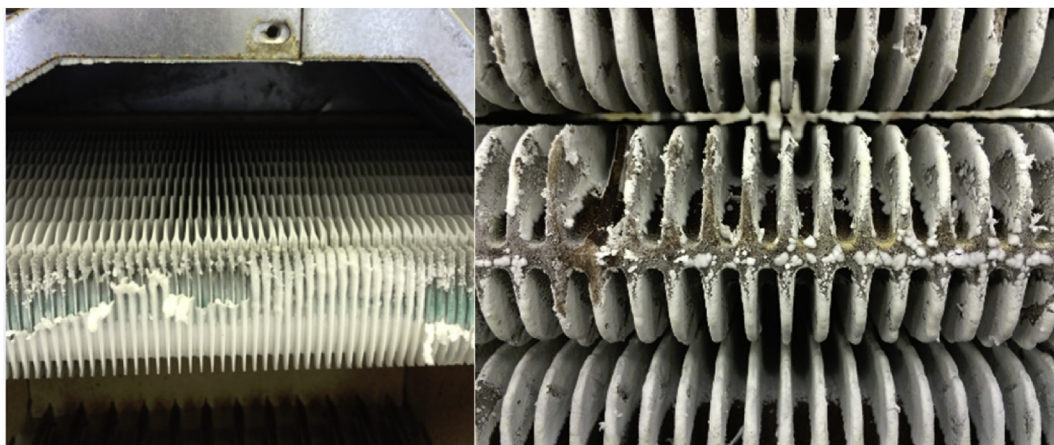
Fig. 4. Left, heat exchanger appliance 2. Right, heat exchanger appliance 3.
