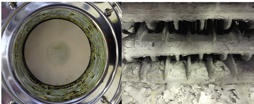
Fig. 7. Silica deposition in the heat exchanger of the appliances 7 (left) and 5 (right) after roughly 1050 h of operation using 11.2 mg Si/m 3 in the fuel.
