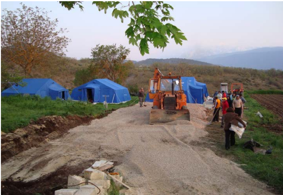
Figure 3.6: The San Giovanni community preparing the foundations for their tent site. Using machinery and gravel provided by some of the residents, here the San Giovanni community prepares the site to which they will move the blue DCP tents. Photo by Sergio Marrone, taken early May 2009.
